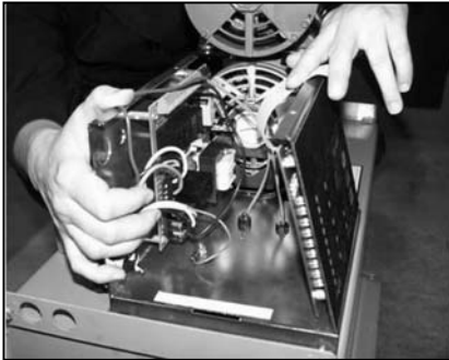
#9 Wires to terminal block
