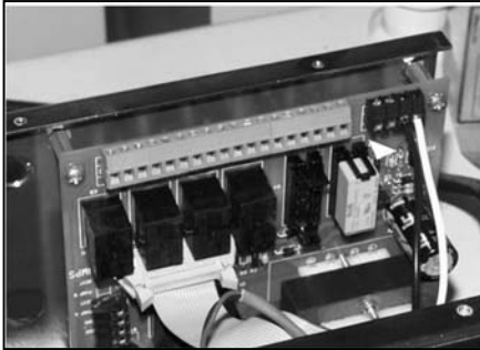
#5 Install critical high relay
