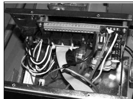
#4 Attach (2) wires from critical high float switch
