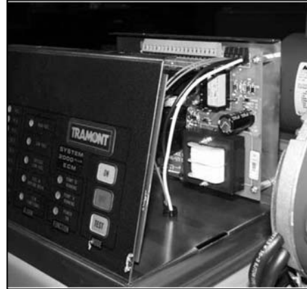
#3 Wires through bottom of ECM
